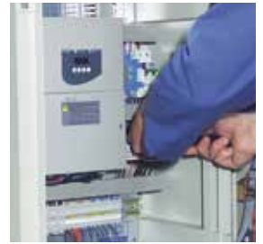
CONTROL PANEL WITH FREQUENCY IN INVERTER
